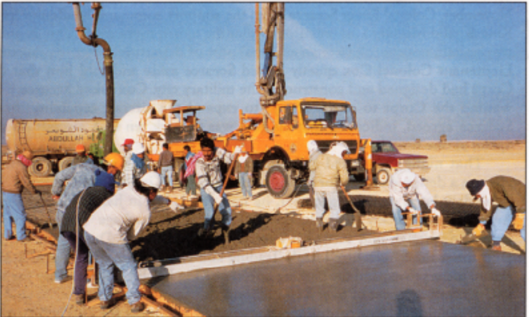
Workers place concrete at one of the four CH-47 helicopter refueling pads. A mechanical screen saved time, allowing the placement of 2,400 cubic meters of concrete in two weeks.
