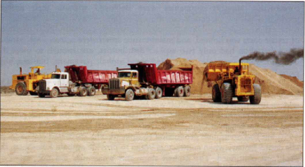
Base course stockpile area for work at KingFahd International Airport. The lack of an adequate source of base course in the eastern province of Saudi Arabia forced contractors to haul material from Abu Hadryiah, 100 kilometers away.
