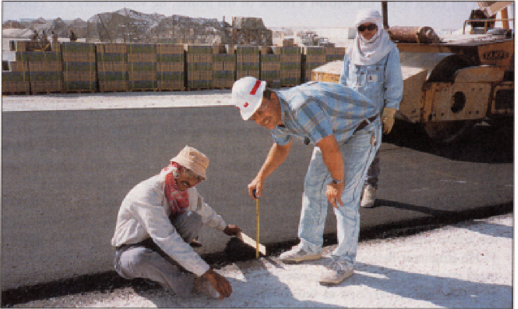
A contractor and Dave Greenwood, Corps representative, inspect the pavement thickness at the Camp Eagle II paving project. Located near King Fahd International Airport, Camp Eagle II was the base camp for the 101st Airborne Division (Air Assault).
